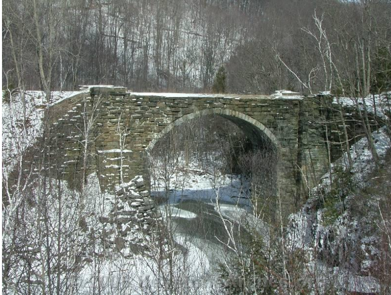
Figure 1. Keystone Arch Bridge This bridge rises seventy feet above the river and is no longer in use by the rail road. 3
